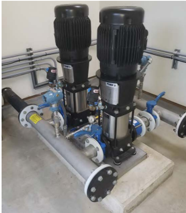
Photo 3 – Oakridge Booster Pumps
