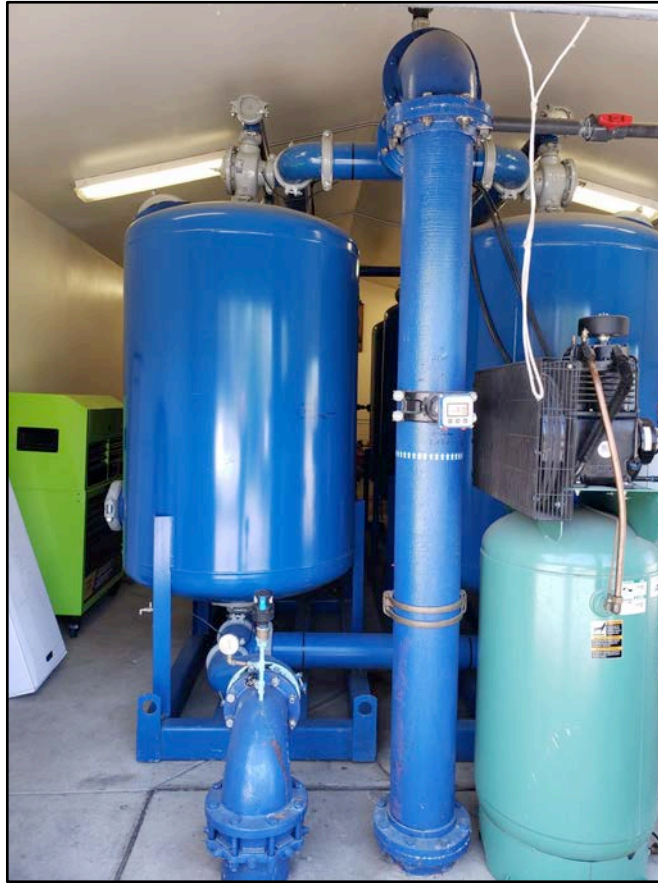
Figure 2-7 Iron and Manganese Treatment System at the San Juan Well
