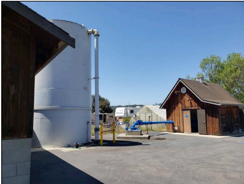
Figure 2-6 San Juan Well and Backwash Reclaim Tank
